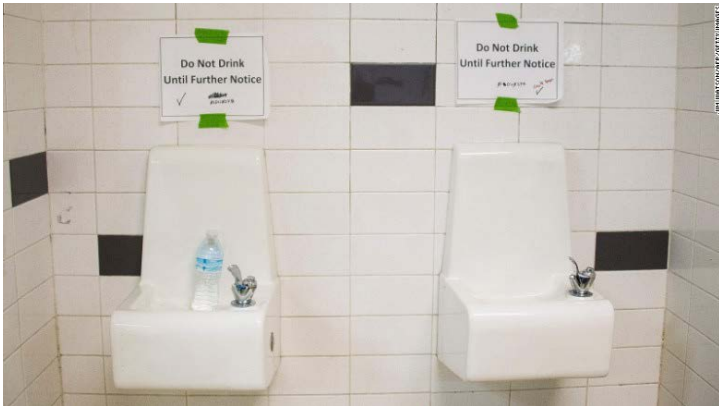
Signs warn against drinking water
