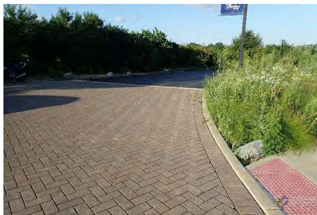
Permeable pavers at the St. Charles Park District's Hickory Knolls Discovery Center driveway and parking lot.
