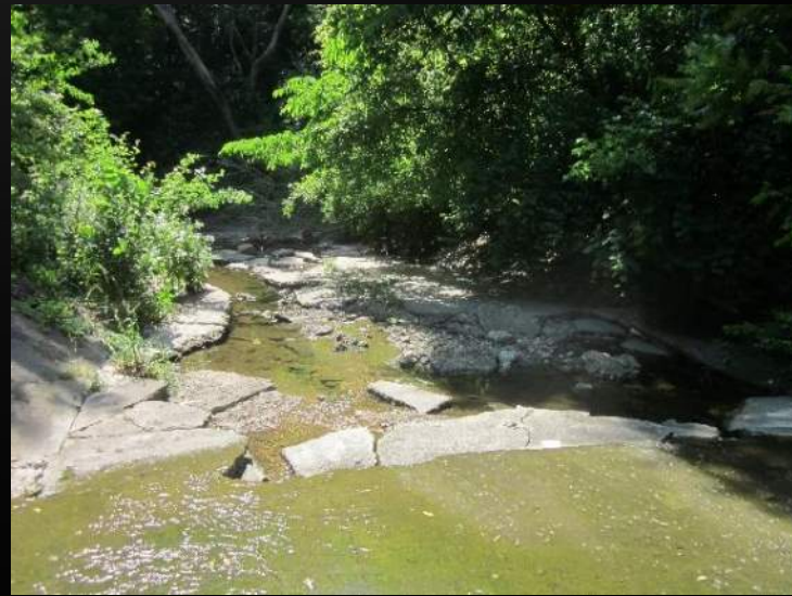
Photo 12: Broken concrete channel
