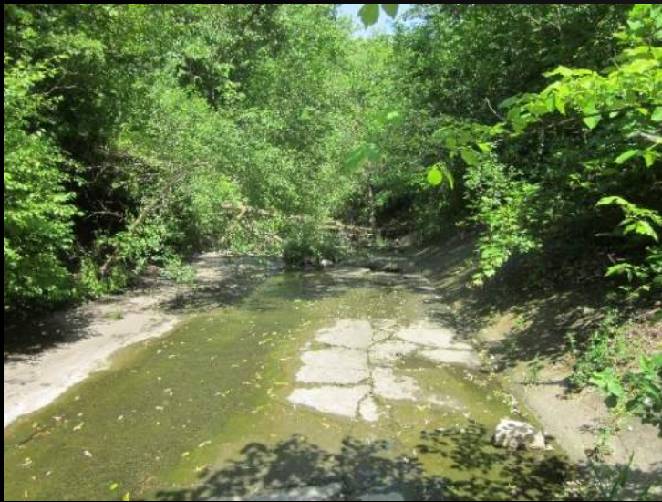
Photo 11: Broken concrete channel, further downstream
