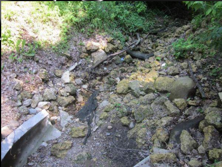
Photo 17: Side channel culvert repair with exposed filter fabric
